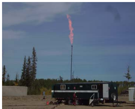
b-002-I Production Testing
